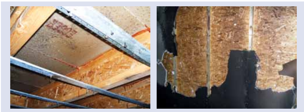
Figure 26 Limited damage to floor joists and party wall. Test F1.
