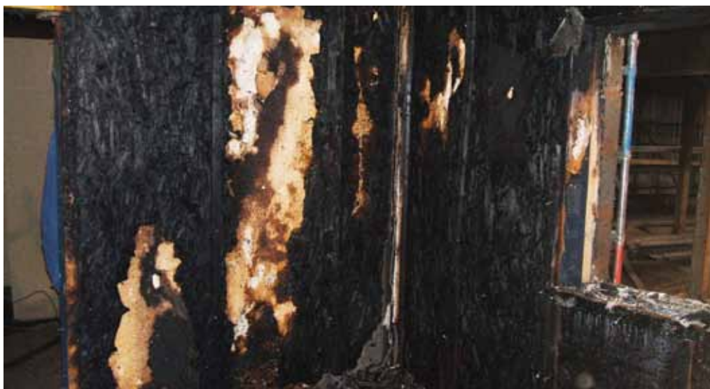
Figure 28 Damage to PUR wall panels. Test F3.
