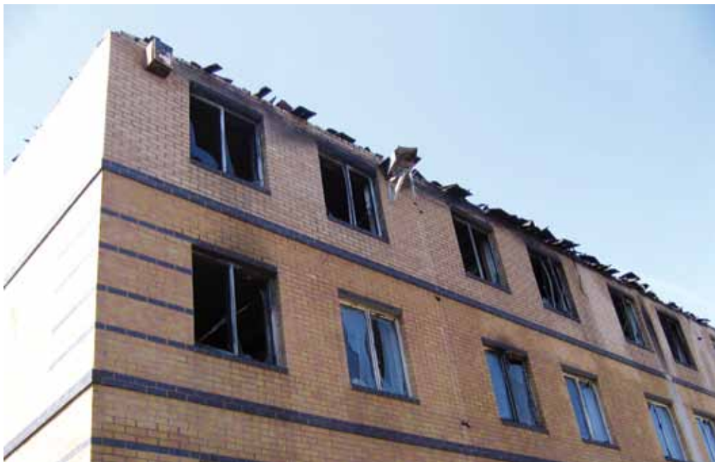
Figure 38 Damage to eastern elevation of student accommodation
