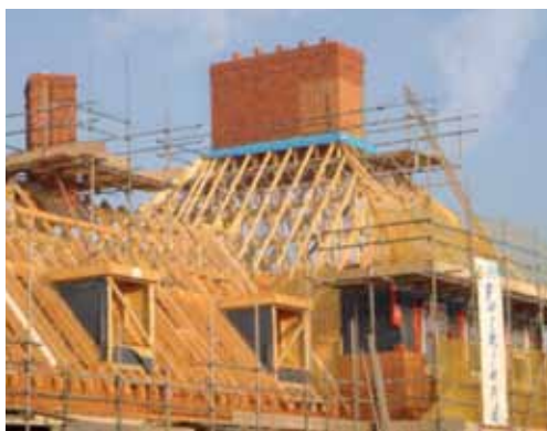
Figure 1 'Mock' chimney breast on a timber frame building (photo courtesy of London Fire Brigade)
