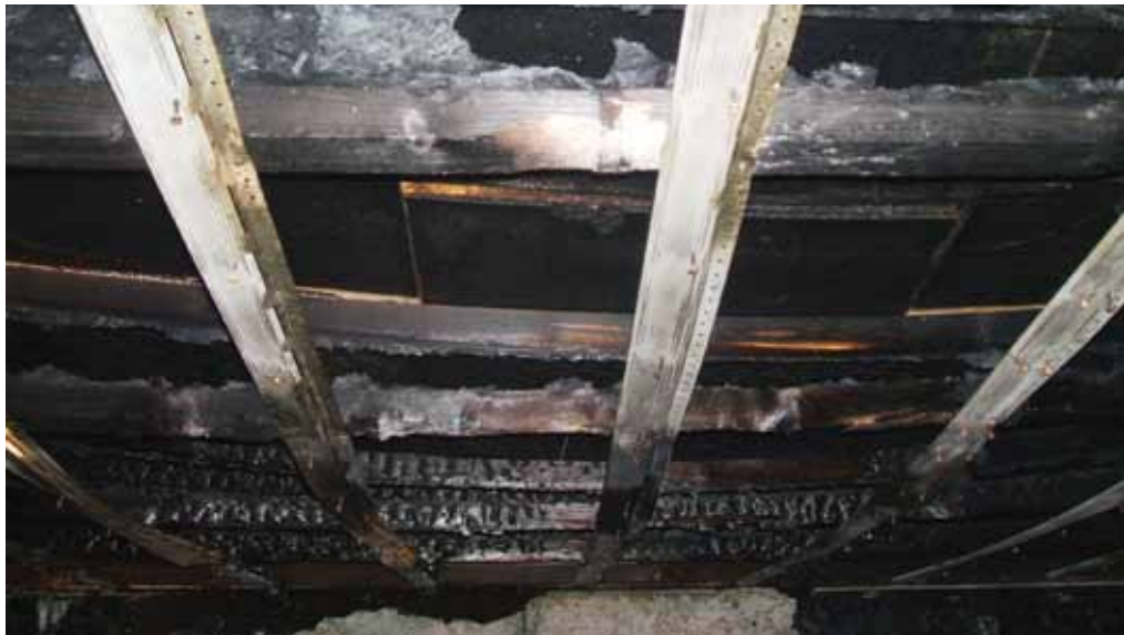
Figure 27 Damage to engineered floor joists. Test F2.
