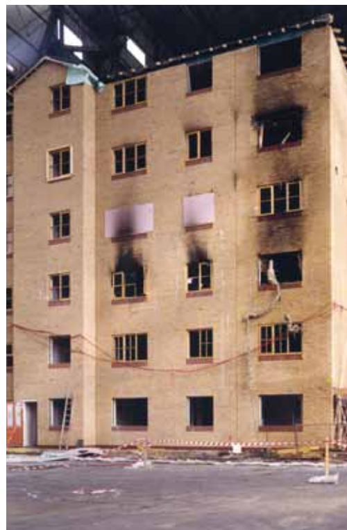
Figure 22 Front elevation of TF2000 building showing extent of vertical fire spread
